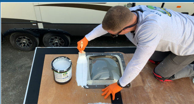
APPLY A THICK AMOUNT OF CRAZY PATCH OVER ALL PENETRATIONS LIKE AROUND SKYLIGHTS
