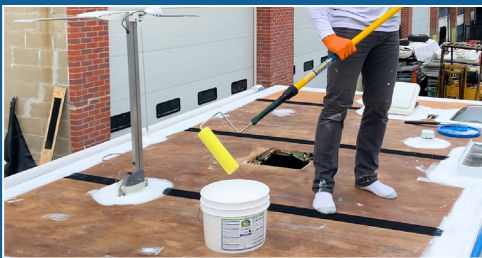
HAVE YOUR ROLLER FRAME READY WITH 1/2" NAP ROLLER ON AN EXTENSION POLE & CRAZY SEAL BASE LAYER
