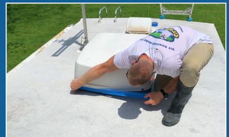
TAPE AROUND AC UNITS
