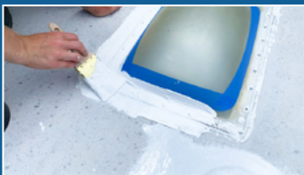
PAINT CRAZY PATCH AROUND SKYLIGHTS
