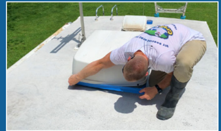
TAPE AROUND AC UNITS
