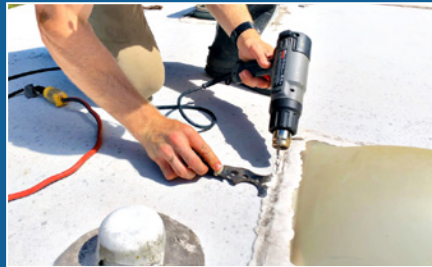
WARMING SEALANT WITH A HEAT GUN CAN HELP
