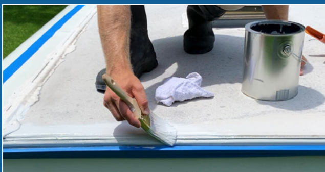
APPLY CRAZY SEAL BASE LAYER OVER CRAZY CAULK WHILE STILL WET. CUT IN SIDES OF ROOF WITH CRAZY SEAL AS YOU GO.
